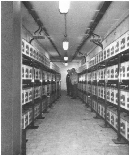
Fig. 13. OGiV 250-Ah energy power battery in a Telecom exchange.
